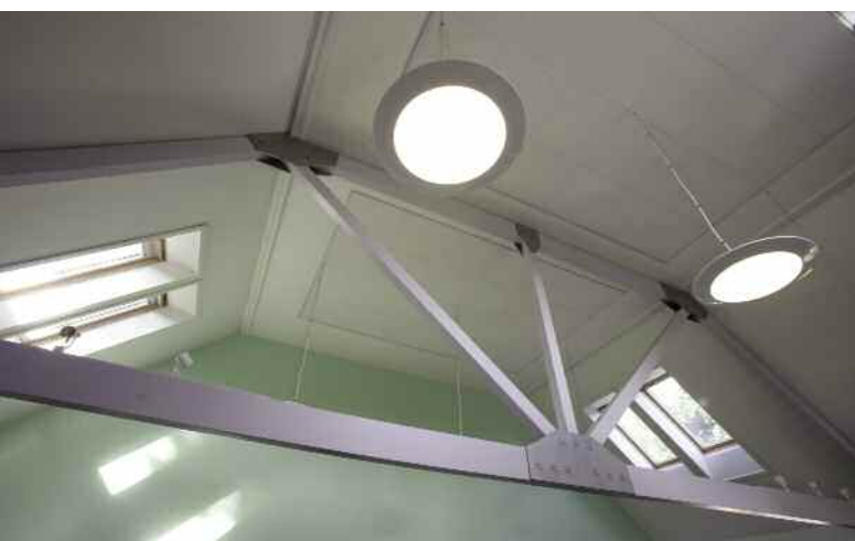
▲ The lighting system fitted by DJA allows the pupils to experience different moods in the main teaching area.
